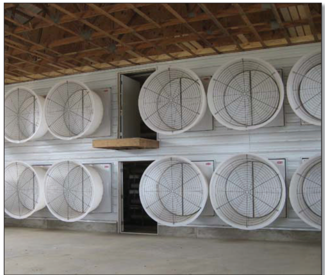
It is advisable to upgrade to tunnel ventilation when a house is converted to enriched colony enclosures. Photo courtesy of North-east Agri Systems
