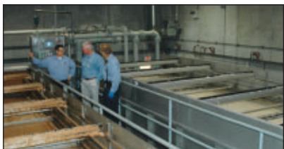
Two stages of dissolved air flotation treatment are employed. Wastewater flows from the primary DAF unit (background) into the aeration basins and back through the secondary DAF unit (foreground).
