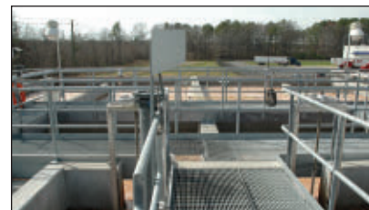
The aeration process features two separate wastewater flow trains (left and right) for flexibility and cross-mixing between anoxic and anaerobic zones (foreground and background) through the use of mixers stationed at port holes in each of the basin's internal walls.
